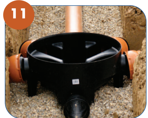
✓ Install inspection chambers wherever there is a change of direction or a junction.
