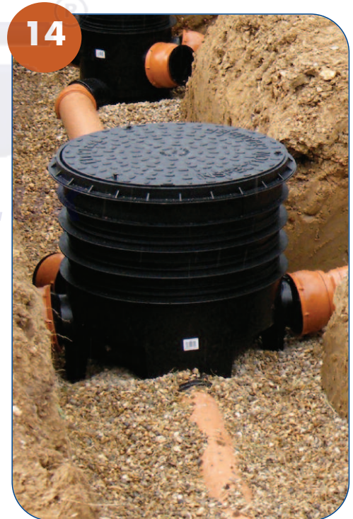
✓ Backfill with pea shingle up to the crown of the pipework, and then backfill using the dug out soil.
